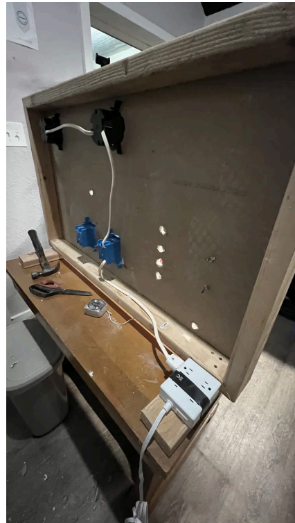
Rear reference — old-work boxes, cable paths, and back-side access before final wiring.
